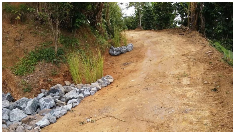
Figure 54. Example of check dams constructed by PDC on a dirt road network in coffee farms of Yauco Puerto Rico.
