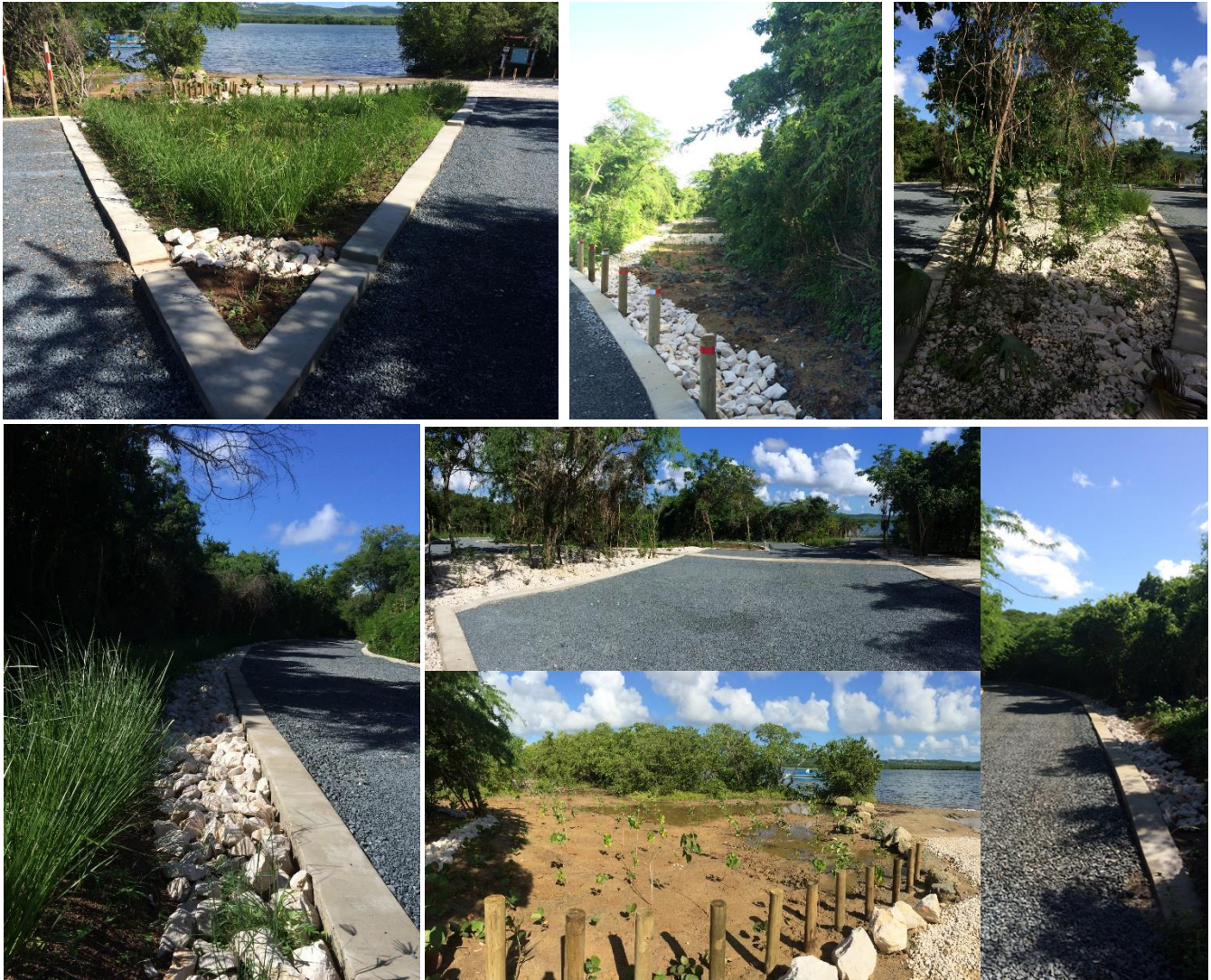
Figure 37. BMPs implemented following a train treatment approach in Mosquito Bay in Vieques Puerto Rico. Practices include bioswale, bioretention, raingardens, constructed treatment wetlands and permeable parking.
