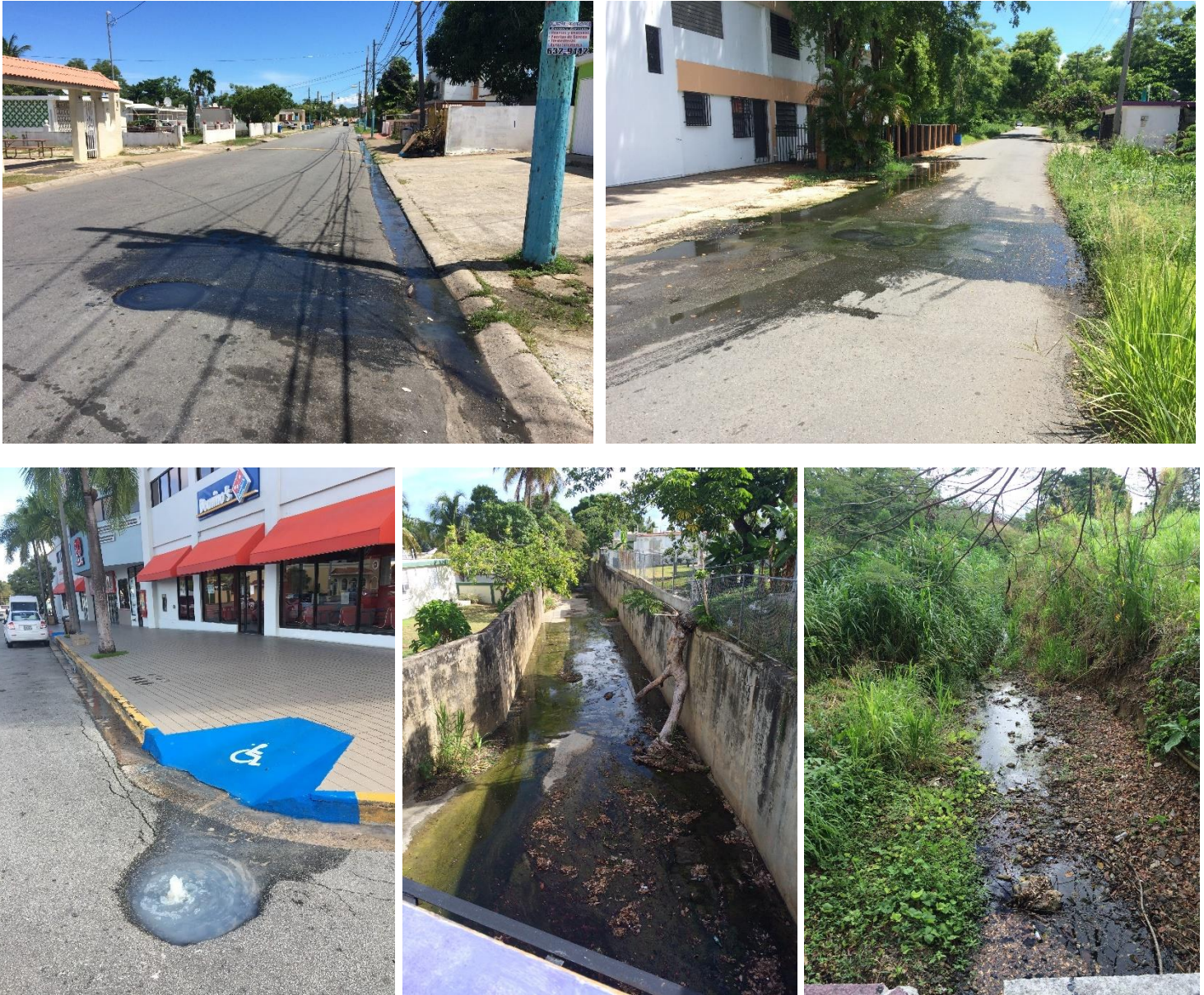
Figure 15. Examples of failing sewer infrastructure across the area. Images provided by Hector Sanchez from the Fajardo Municipality Planning Board and PDC staff. Pictures are from 2014, 2016 and 2017 showing persistent problems of sewage overflows.
