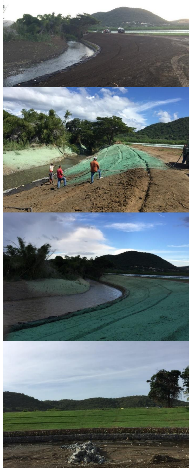
Figure 52. Hydroseeding implementation by PDC on a riverbank stabilization project in the Río Loco, Guánica Puerto Rico
